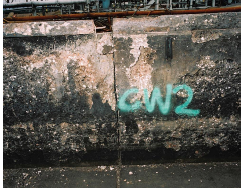
Dislodged bund capping after Buncefield fire
